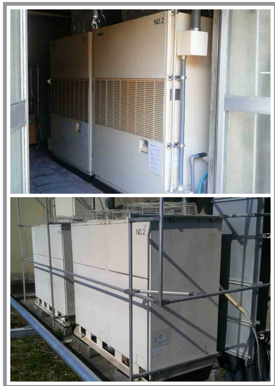
Before replacement Air conditioners of electric package type
