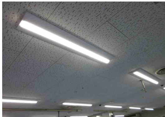
After replacement LED
