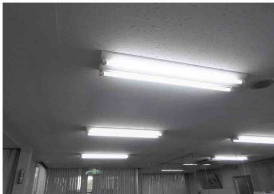
Before replacement Fluorescent Lamps
